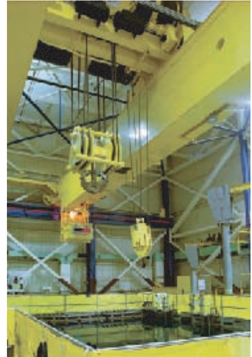
125 Ton Nuclear Fuel Handling Crane
