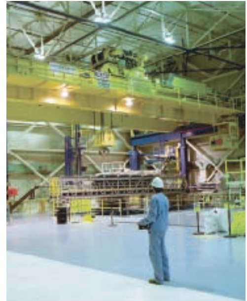
Cask Handling Crane
