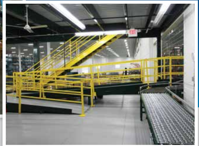
Custom catwalk and ramp designed to connect new mezzanine to existing mezzanine in adjacent building.
