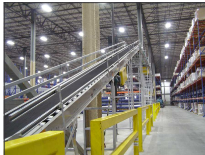
Conveyors & High Bay Storage
