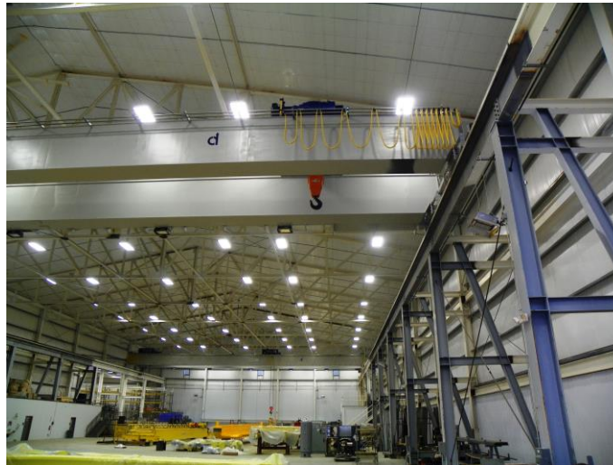
Two (2) 50 Ton Top Running Double Girder Cranes
