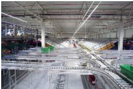
Picture 5: The conveying technology transports the totes to the workplaces.
