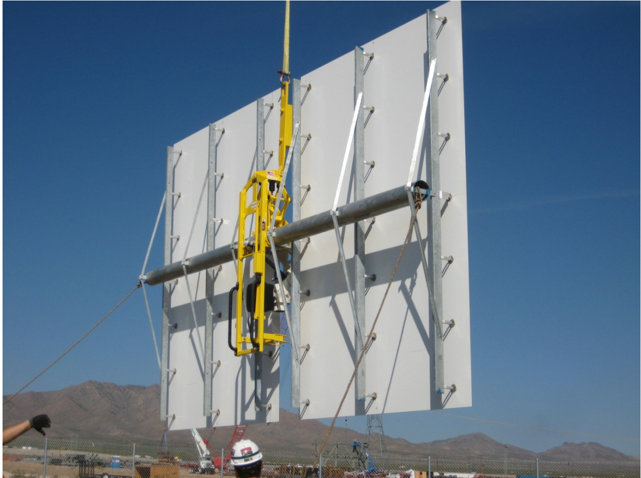
Bushman Heliostat Reflector Lifter being used to set a reflector into its pylon at the Ivanpah Solar-Electric Generating System being constructed in Nipton, CA.
