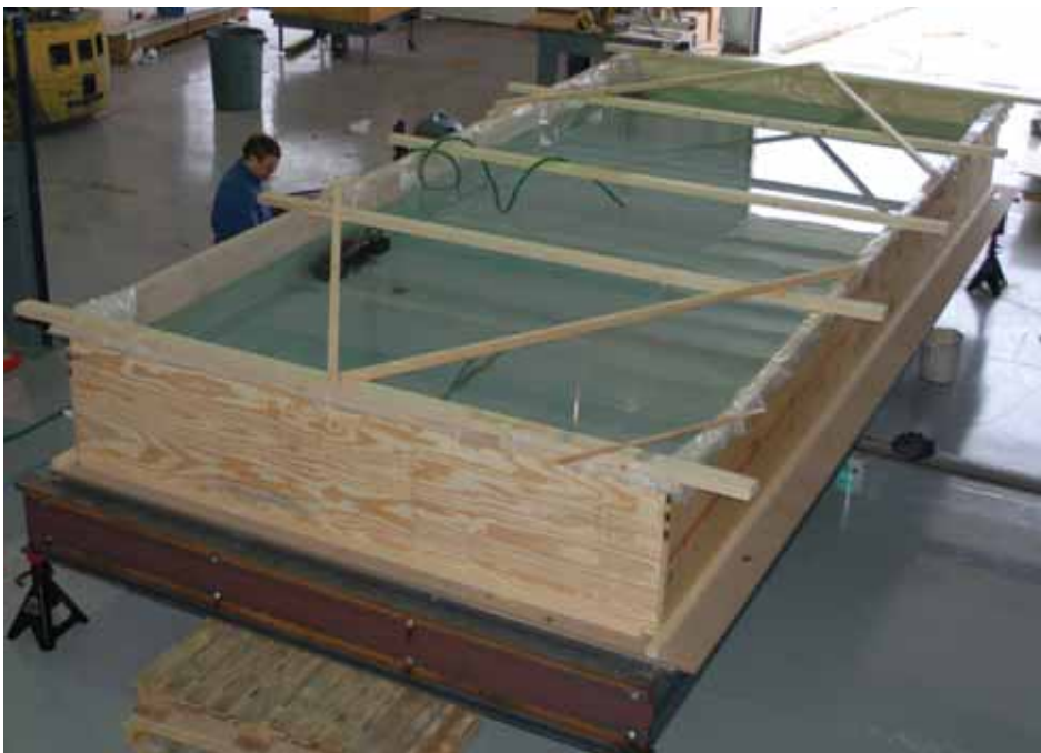
Cornerstone Specialty Wood Products recreates a uniform loading condition on a large platform.
