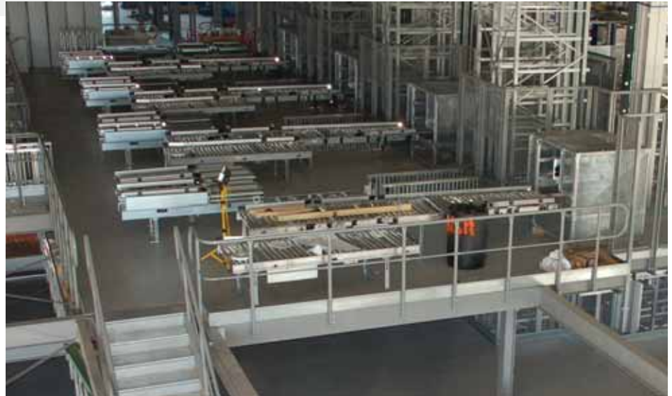
130,000 square feet of ResinDek LD50 installed at a Warehouse Distribution Center in Canada.
