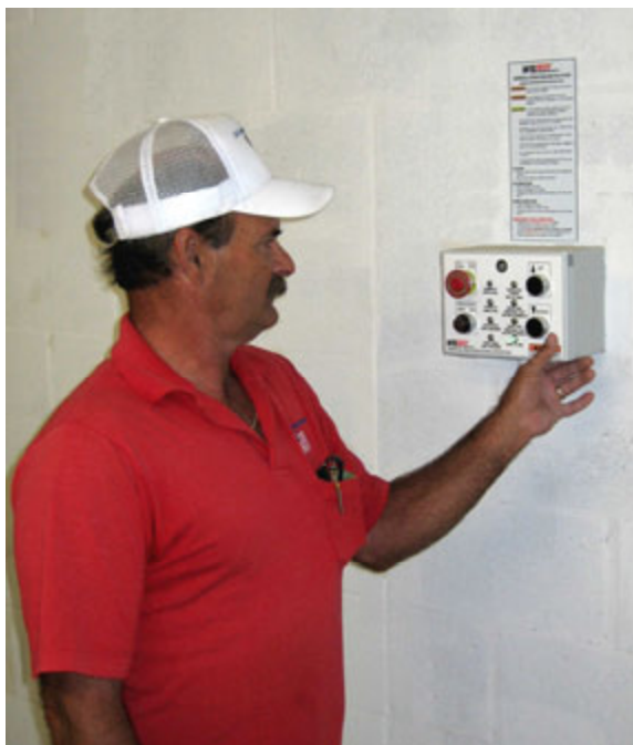
Jim Gearhart operates Wildeck's user-friendly EZ-Pro VRC control. Clearly marked buttons and bright LED lights instantly signal lift status and inform the operator when the lift has been off-loaded for return to ground level.
