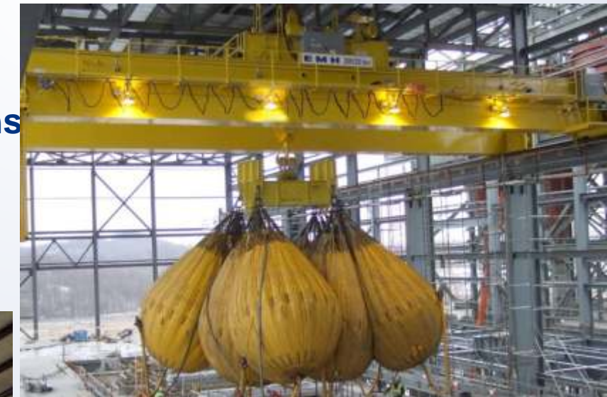
A 250/50 ton engineered crane undergoes load testing at a power plant. The specially engineered hoist at right features a service walkway to facilitate maintenance.
