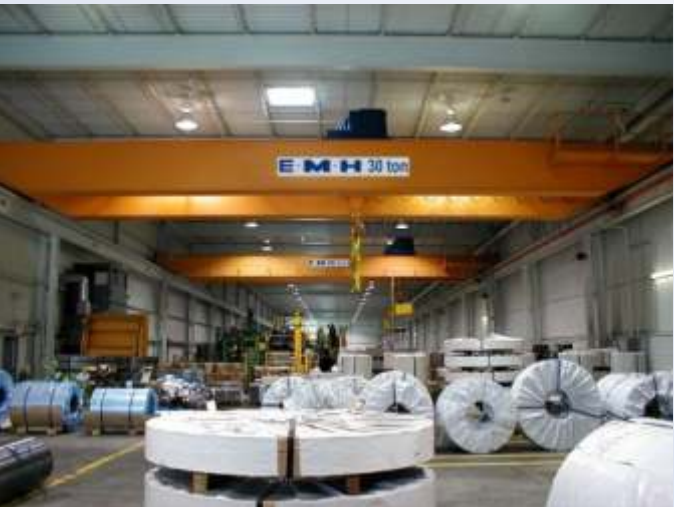
Two 30 ton EMH cranes with engineered hoists move large coils for two shifts each day at an Ohio steel service center.
