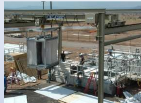
A NOMAD Free Standing Crane system is used outdoors at this western water treatment plant. The crane lifts and changes filters.
