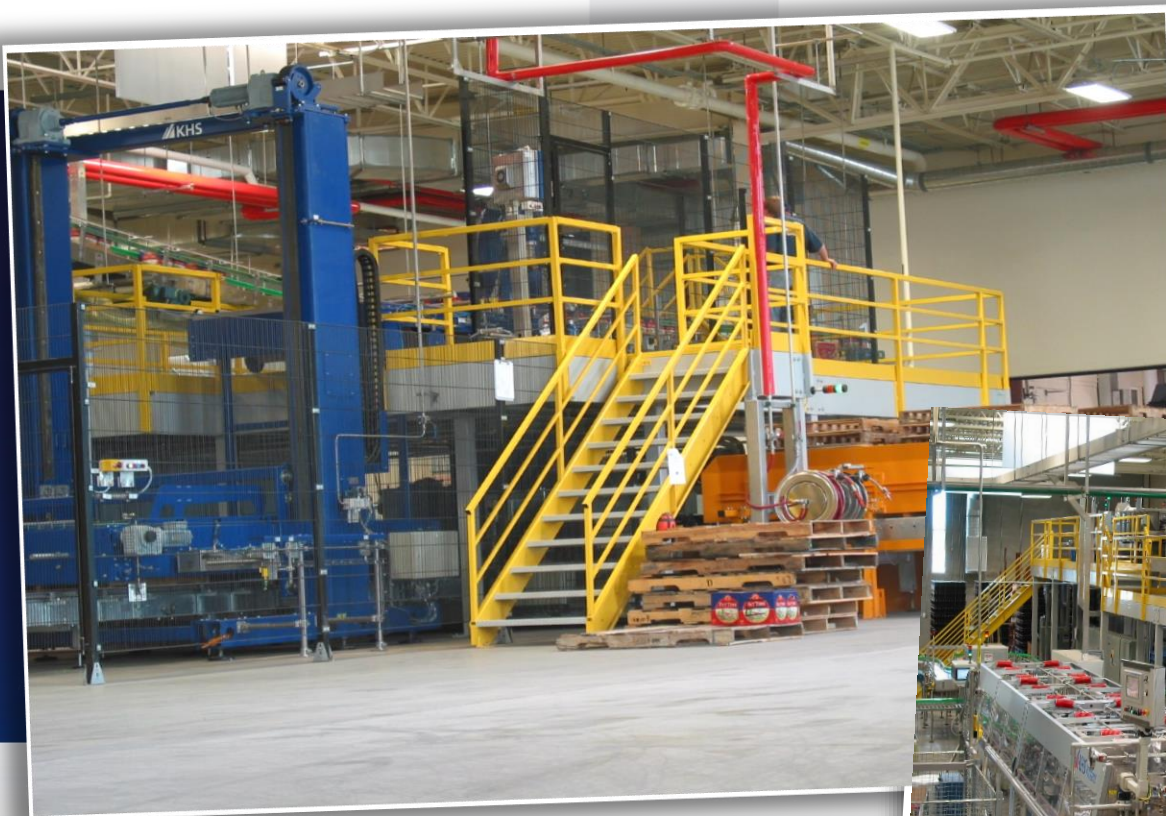
Overhead platform wraps around case palletizer allowing access to equipment.
