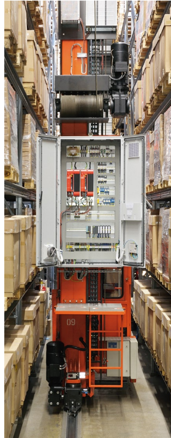
After just three days of conversion work and testing this storage and retrieval machine, which now has a S7-switch cabinet and new driving and hoisting drives, was again ready for immediate use.
