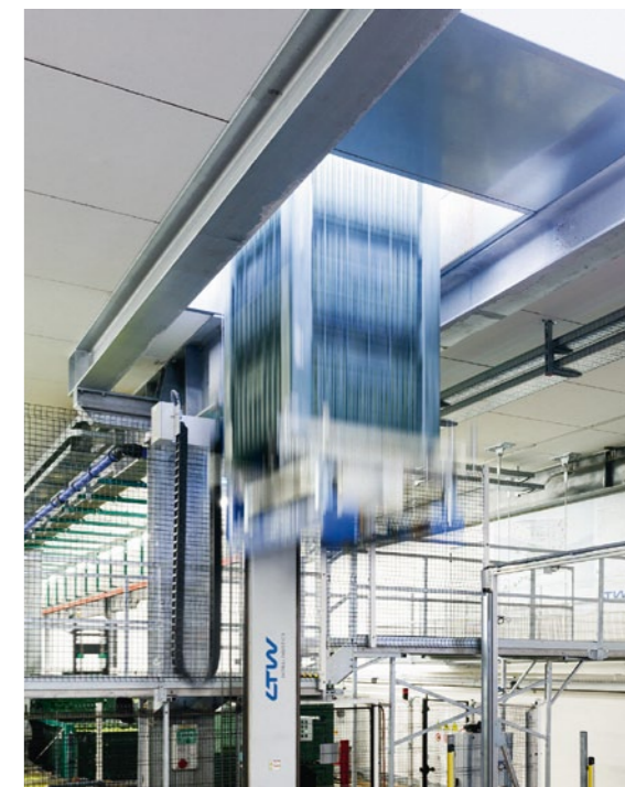
The two-storey, automatic conveyor system between the sorting system and the high-bay warehouse with two transfer cars (top picture) and two vertical lifts (bottom picture).
