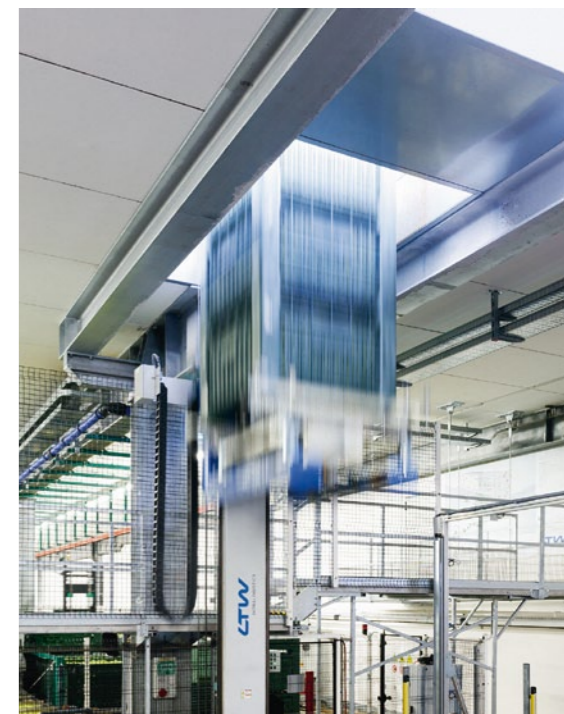
The two-storey, automatic conveyor system between the sorting system and the high-bay warehouse with two transfer cars (top picture) and two vertical lifts (bottom picture).
